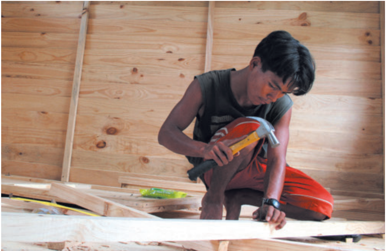
As part of the American Red Cross transitional shelter program, residents in Aceh, Indonesia, still rebuilding after the 2004 tsunami, do hands-on work in the assembly process.
